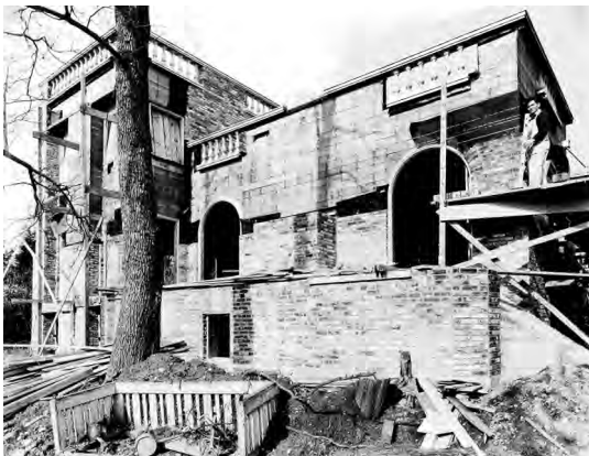
Dr. Cecil L. Tenny's home under construction in the 1900 block of Magnolia Boulevard West in the early 1930s.
