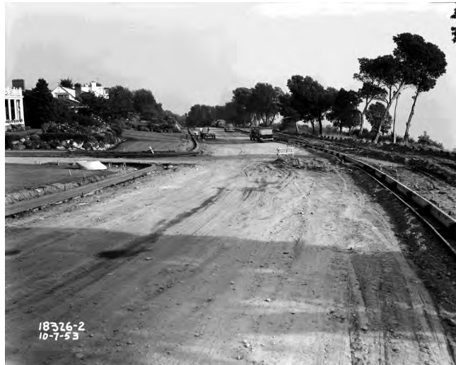
Road work widening Magnolia Boulevard West. Seattle Municipal Archives, Engineering Department Photographic Negatives, #44547. October 7, 1953.
