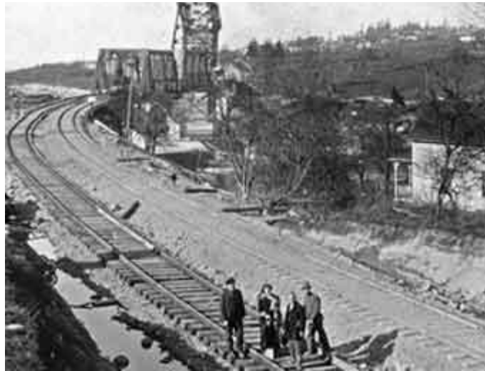
Finishing the Great Northern Train Bridge, the Magnolia side looking toward Ballard. Circa 1913. Courtesy of Paul Dorpat.
